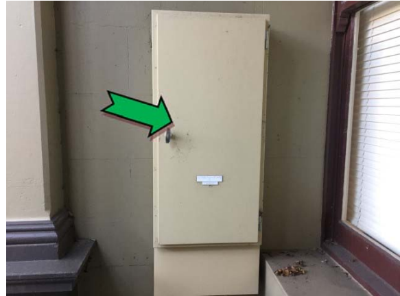
Photo 2. Exterior, west elevation, electrical backing board – suspected non asbestos-containing bituminous backing board.
