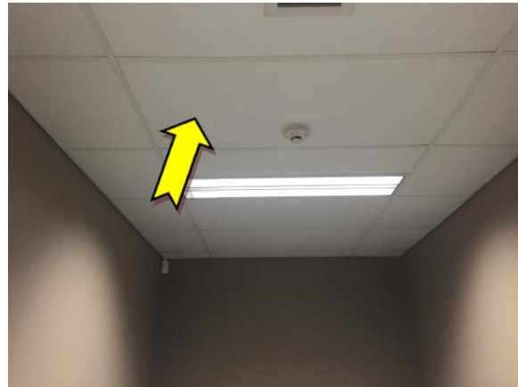
Photo 16. Interior, ground level, toilet, ceiling – suspected SMF compressed ceiling tiles.
