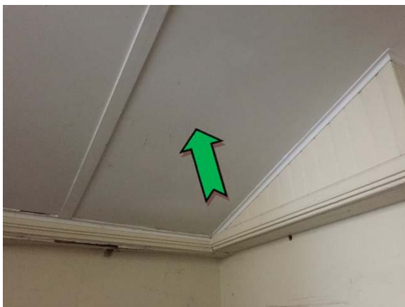
Photo 5. Interior, level one, corridor, adjacent disabled toilets, ceiling – suspected non asbestos-containing fibre cement sheeting.
