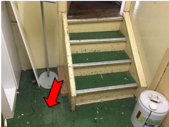
Photo 9. Interior, level one, storeroom, floor coverings – asbestos-containing vinyl floor tiles.
