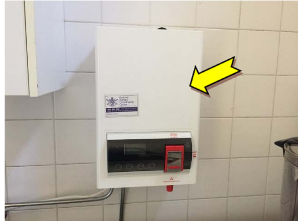
Photo 14. Interior, level one, kitchen, hot water boiler – suspected SMF internal insulation material.
