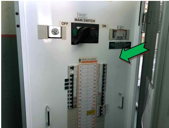
Photo 3. Interior, level one, west elevation, corridor, electrical backing board – suspected non asbestos-containing bituminous backing board.
