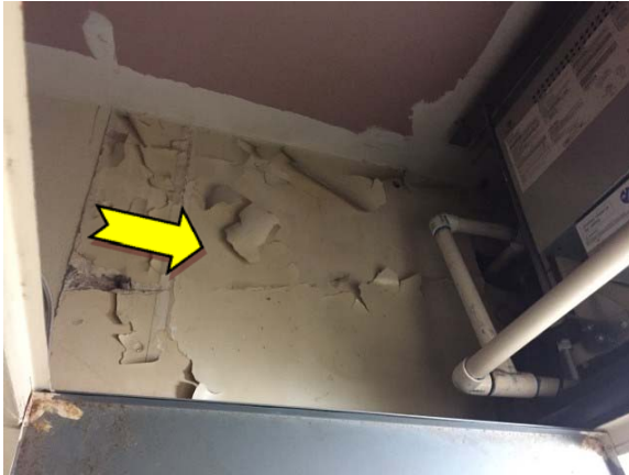
Photo 19. Interior, ground level, throughout, ceiling space – lead-containing cream upper paint systems.
