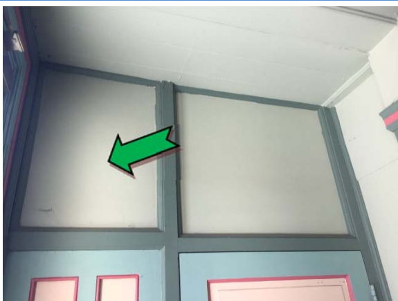
Photo 11. Interior, ground level, north-east elevation, above cupboard, infill panel – non asbestos-containing fibre cement sheeting.
