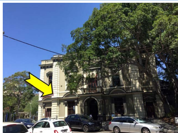
Photo 18. Exterior, throughout, features – suspected lead-containing cream upper paint systems.
