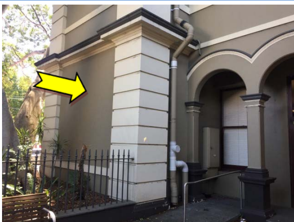
Photo 17. Exterior, throughout, walls – lead-containing white lower paint systems and suspected lead-containing green upper paint systems.
