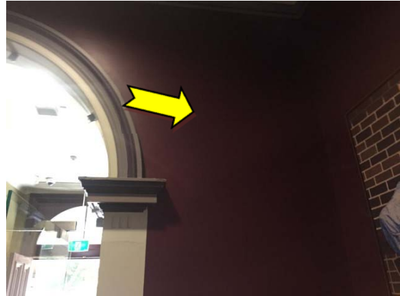
Photo 20. Interior, ground level, entrance, walls – suspected lead-containing red and light green upper paint systems.
