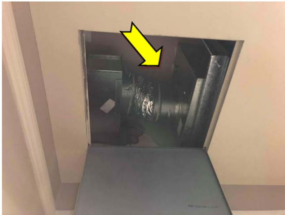
Photo 15. Interior, ground level, ceiling space, throughout, ductwork – suspected SMF internal insulation material.
