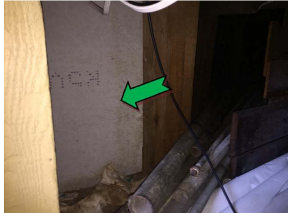
Photo 8. Interior, level one, main hall, beneath stage, wall – non asbestos-containing fibre cement sheeting.
